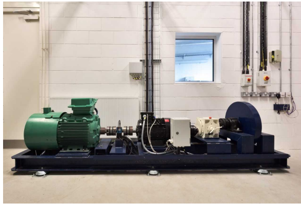
Figure 15. Experimental setup: the rotatory emulator connected to the microgrid at UCC, courtesy, MaREI facility [59].
